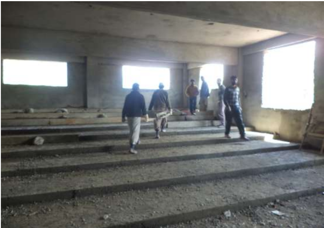
Cement concreting work in progress in one of the class rooms in Ground floor
