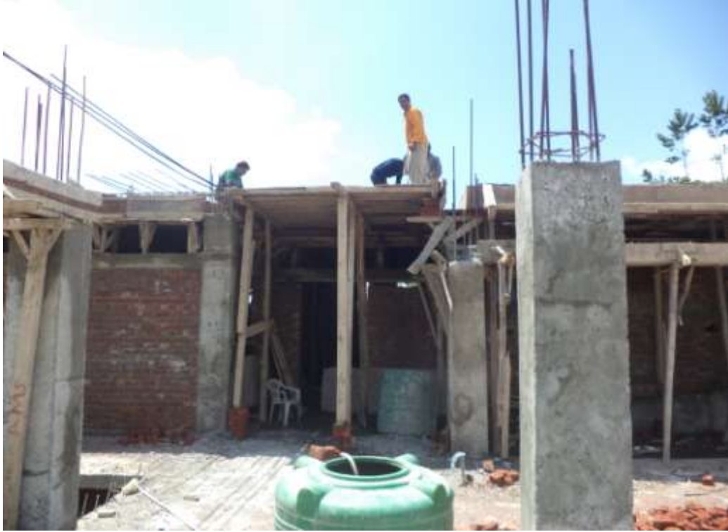
(Right Wing) - Scaffolding work for laying of slab of first floor underway
