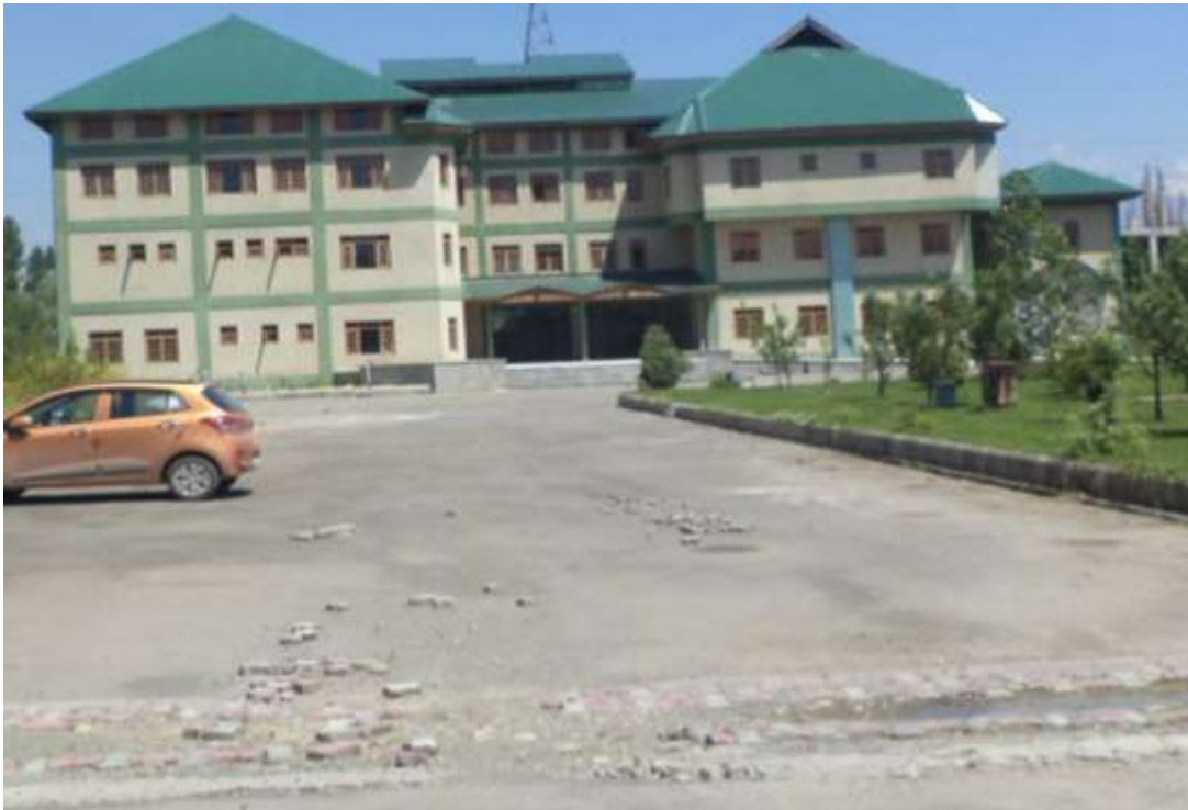
Front view of Residential Block and portion of damaged walkway
