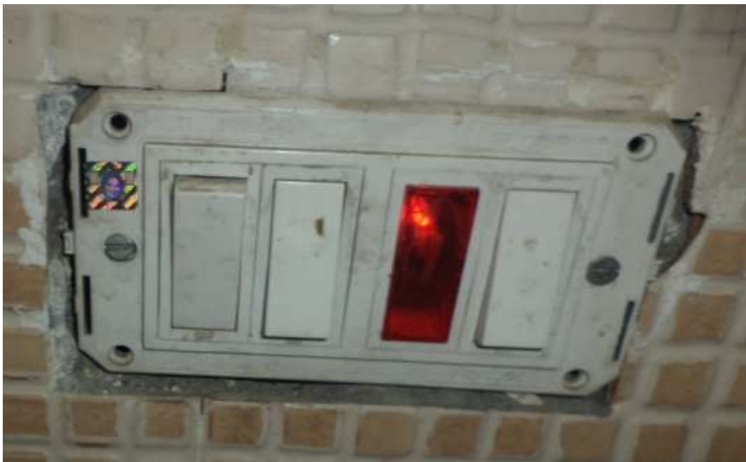
Damaged electric switch plate in one of the rooms of CFC building
