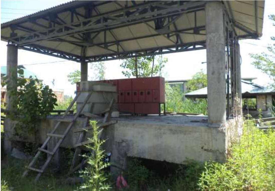
Installation of AVR (63 KVA capacity) within the premises with cables floating in water beneath the platform
