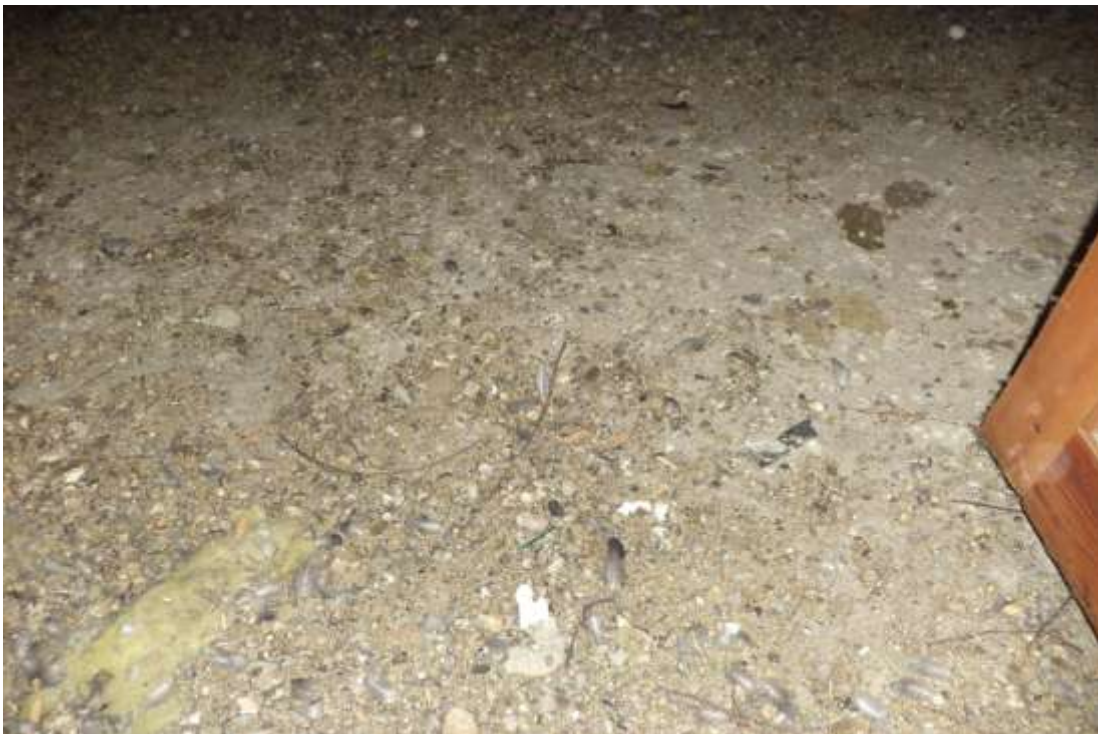
Floor littered with bird droppings and feathers within the building
