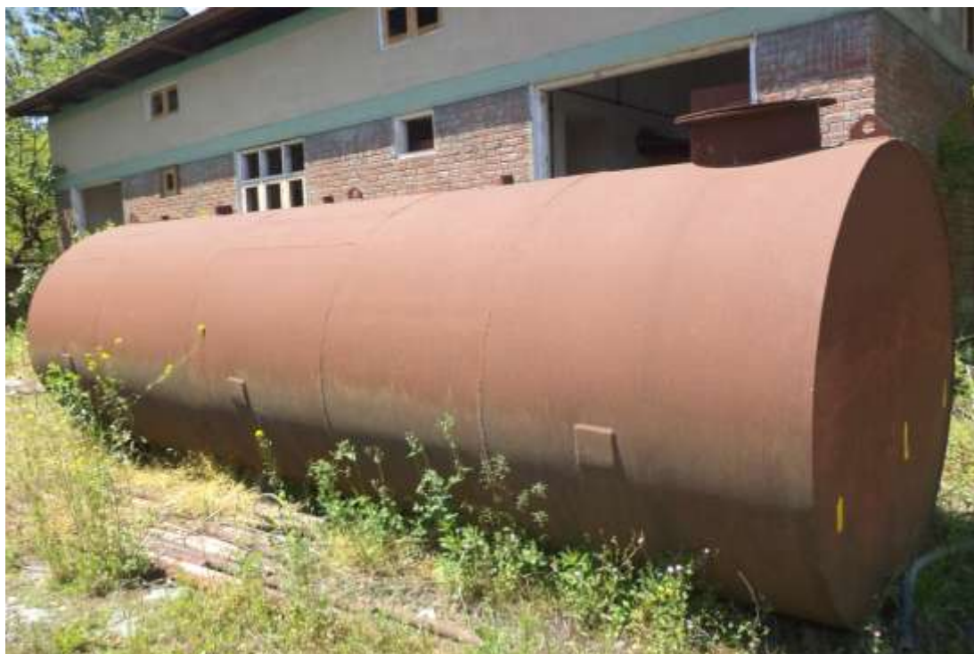
Structure constructed for Boiler room and oil tank of 15000 ltrs capacity grounded within the premises.
