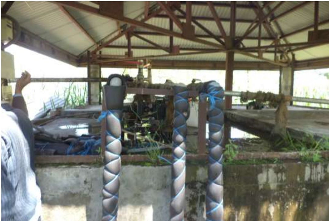
Water sump with capacity of 12000 Ltr constructed within the complex
