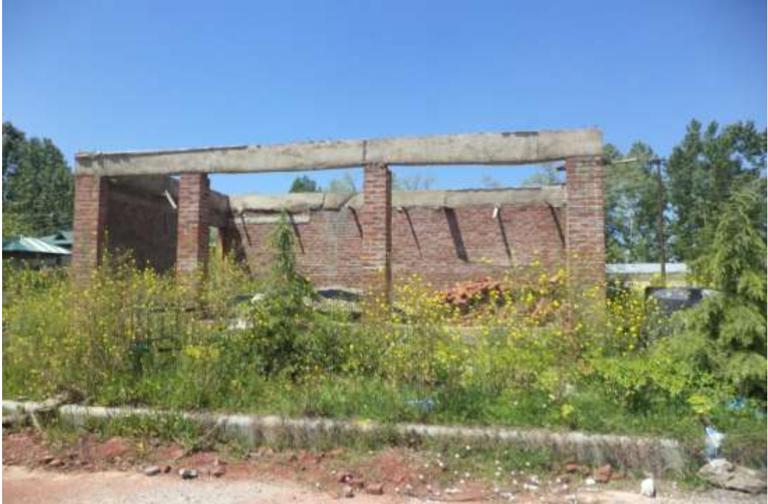
Abandoned Market/ Health centre in Haj House complex
