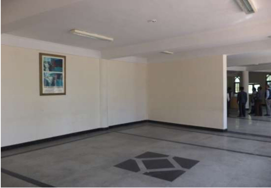
Granite flooring provided in circulation areas of Ground Floor of CFC
