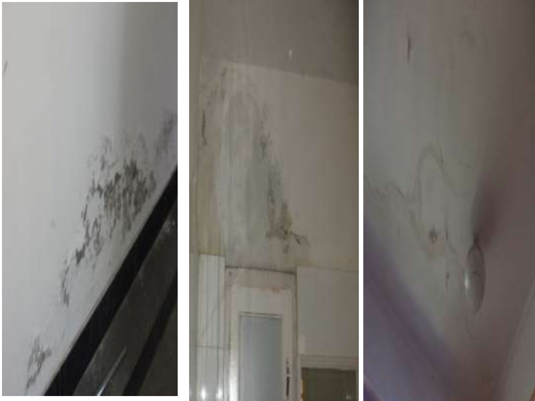
Damaged/ cracked PoP Ceiling in few of the rooms in building blocks
