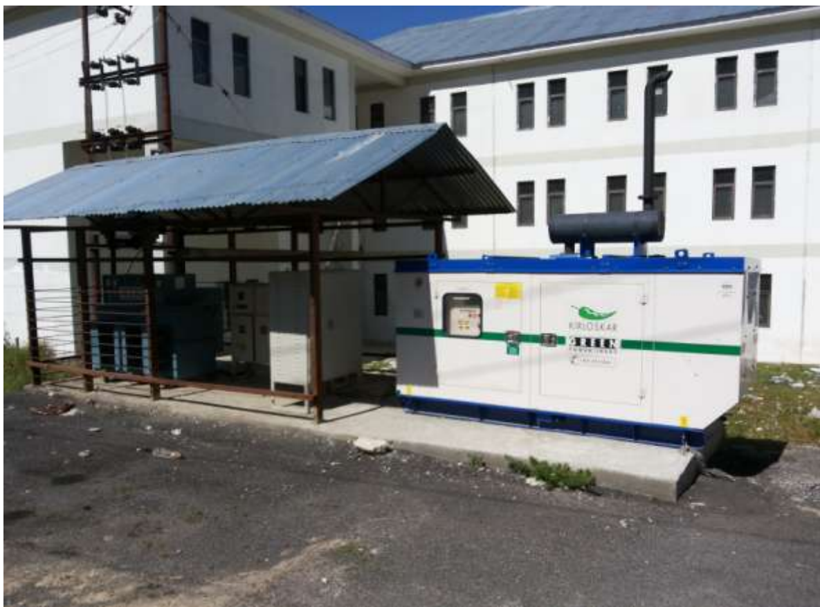
Electric Power Generator and Control Panel
