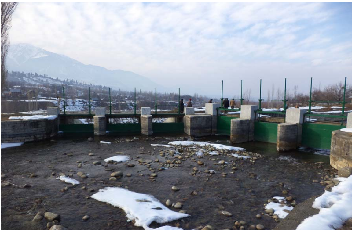
Head regulators for Ahaji canal near Arizal
