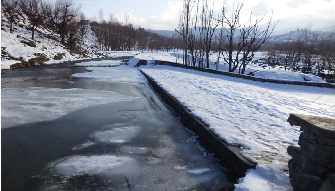
Escape constructed for overflow on the supply channel of Ahji canal near Arizal
