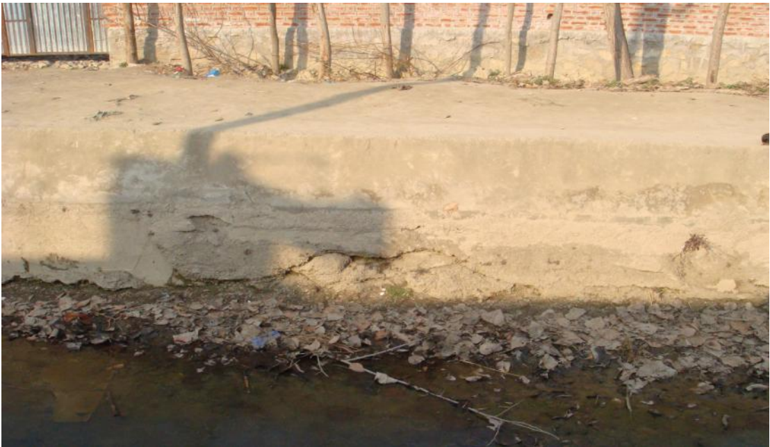
No sign of sidewall/laying of bed treatment
