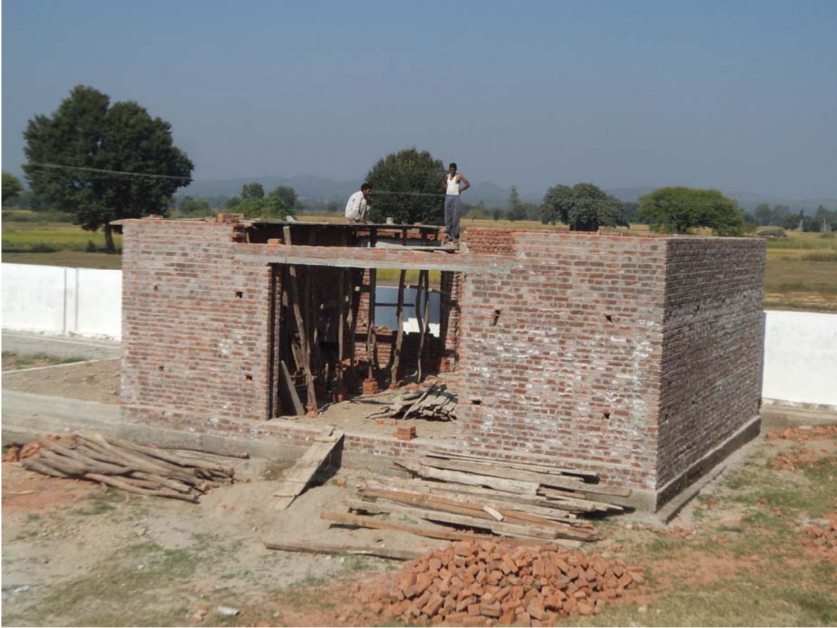
Electricity control room
