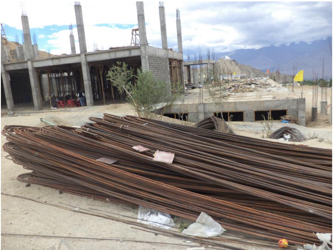
Tar steel dumped at project site
