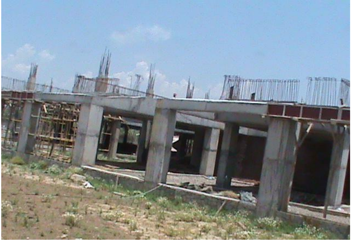
Side view of the N 2 block
