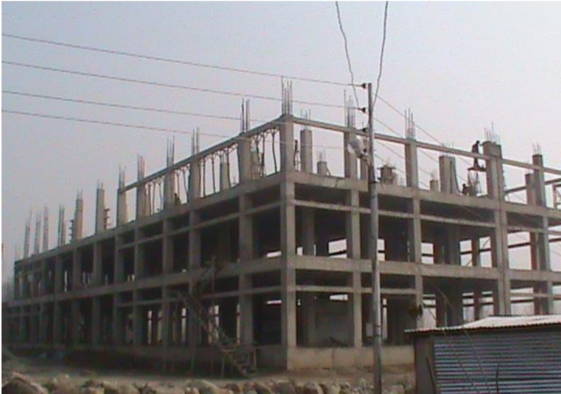
Block C – Slab over 1 st floor completed, Column structures for 2 nd floor in progress
