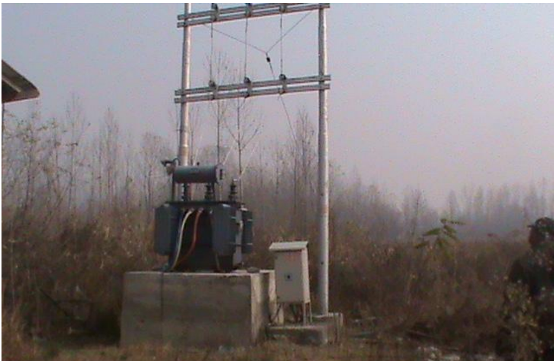
Electric sub station of the capacity of 250KVA installed within the premises of Hospital
