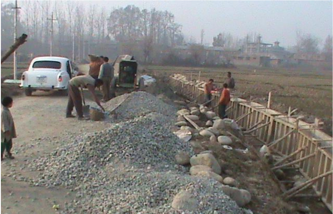
Construction of concrete edge wall and side drain along the approach road
