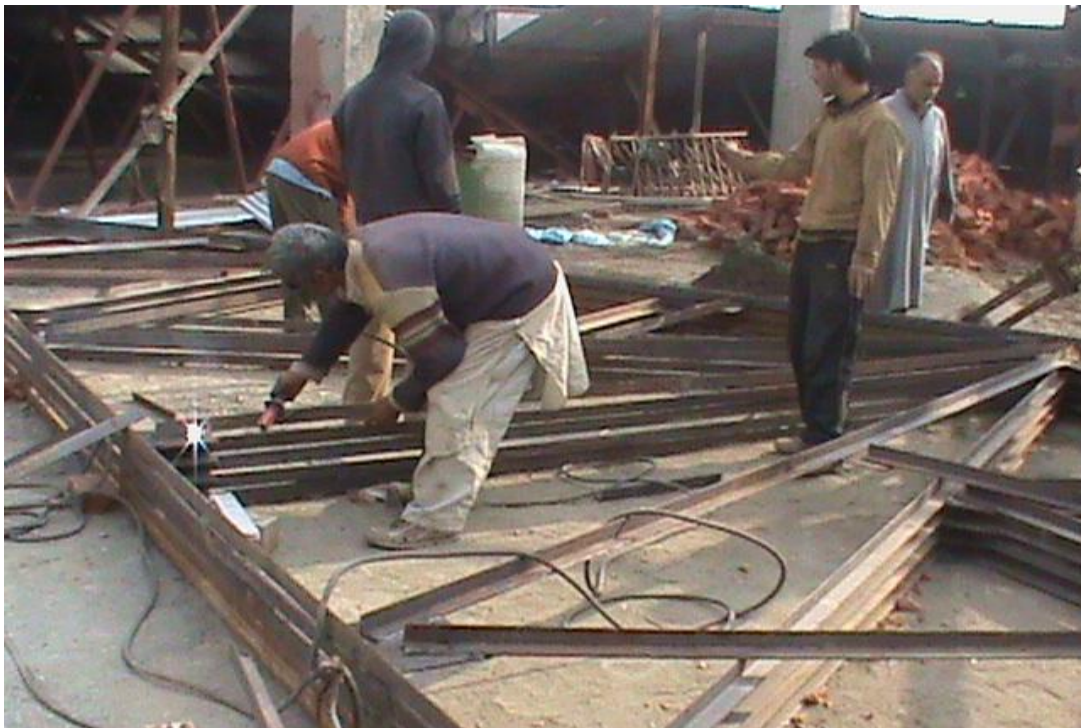
Work of installation of steel truss on top of Middle portion underway
