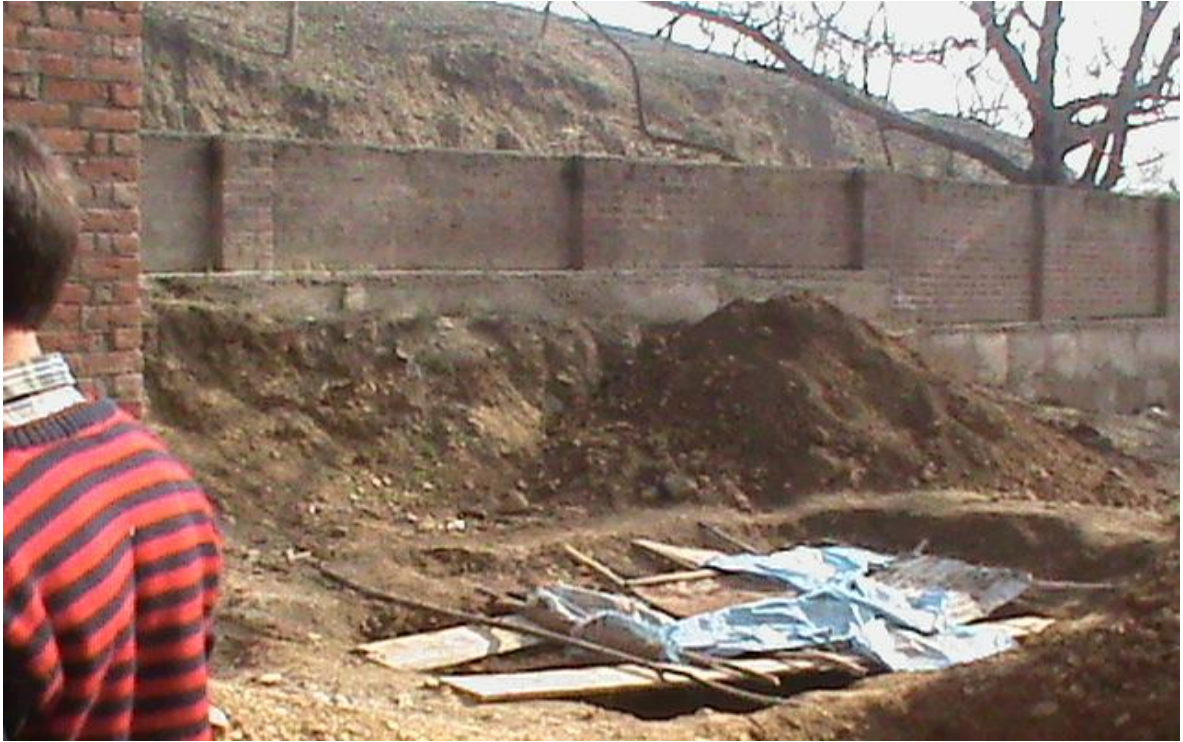
Boundary wall on main road side which requires increase in the height
