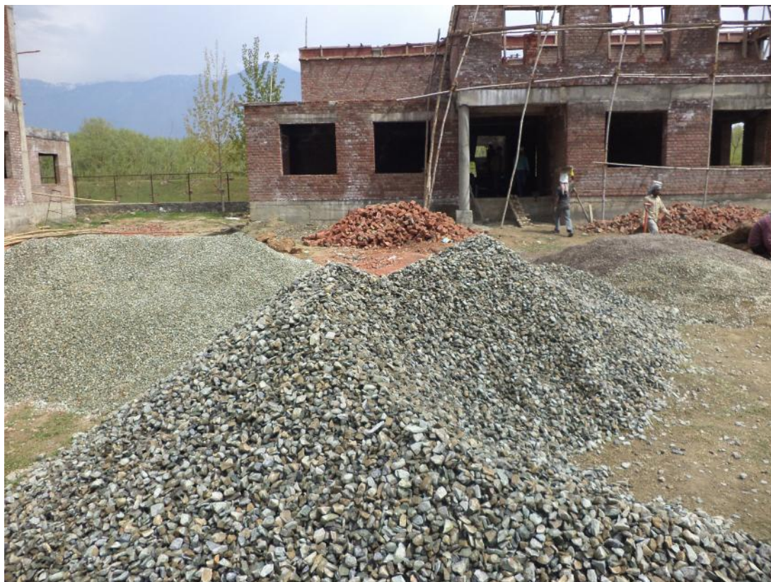
Construction material dumped at site
