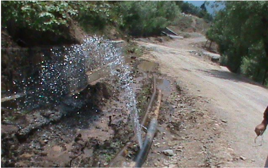
Water supply pipes leaking on the road side
