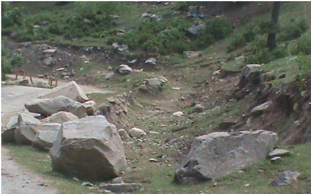
Irrigation canal under construction on Km 14 th on the uphill side of the road.
