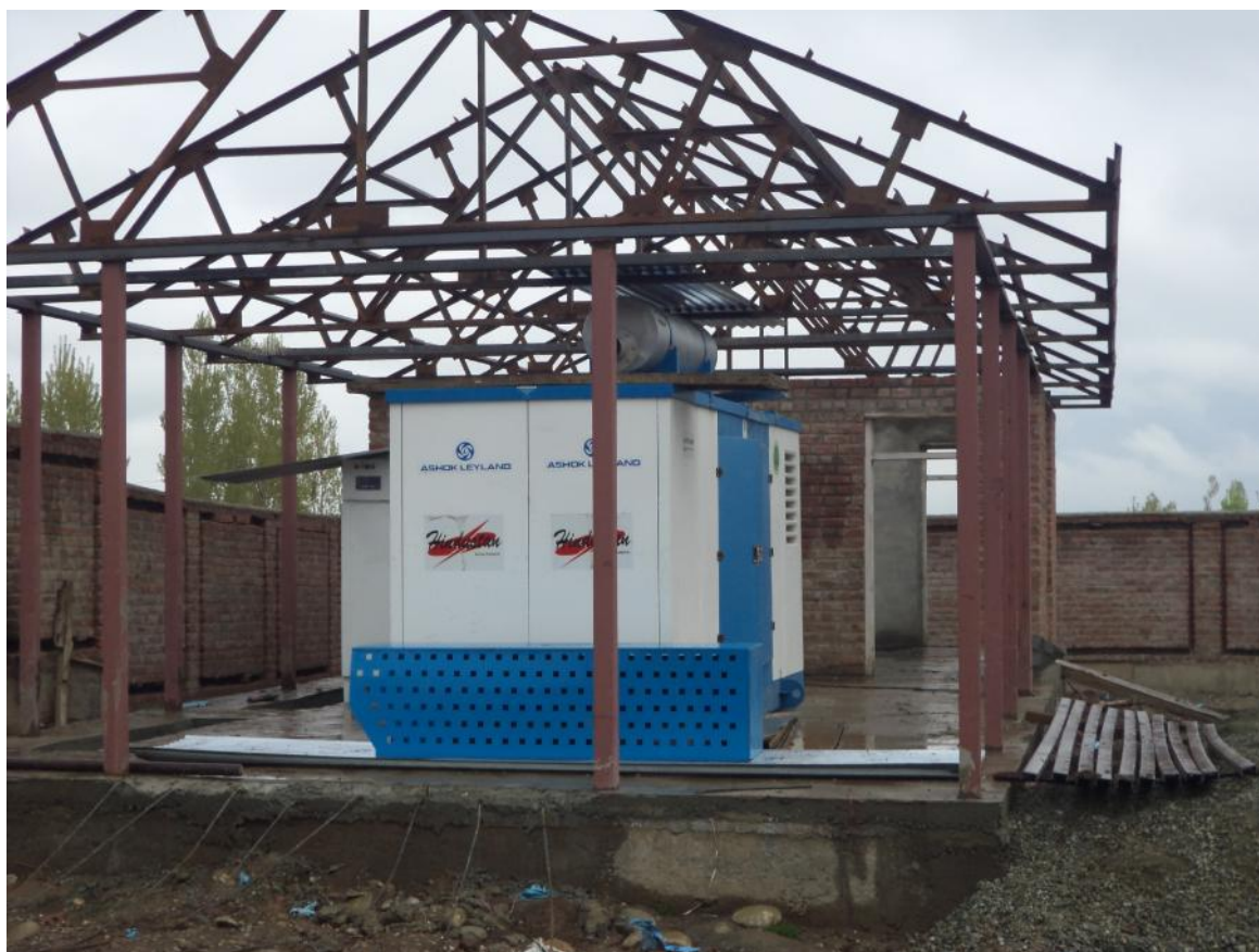
250 KVA DG set installed
