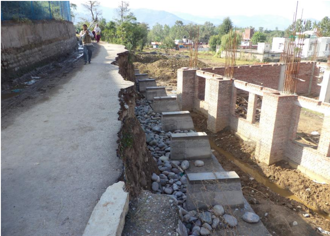
View of eastern side where protection work is further required to safeguard the road
