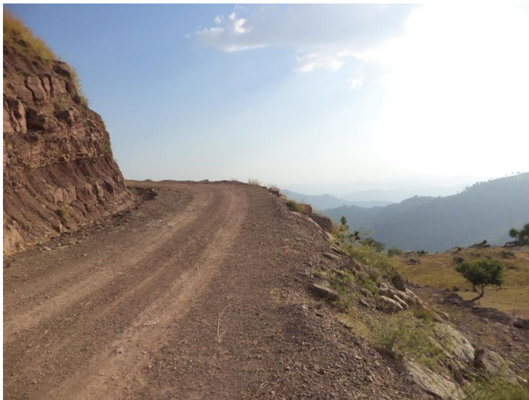
One of the spots where protection work is required
