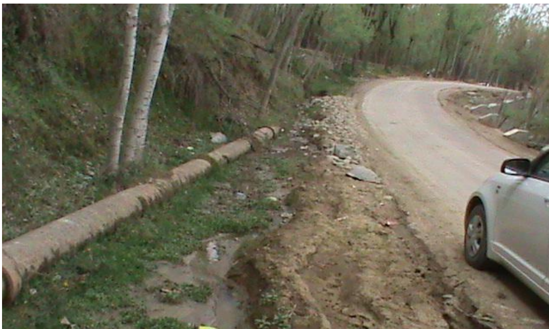
View of the messy and jumbled earthen berms of the road
