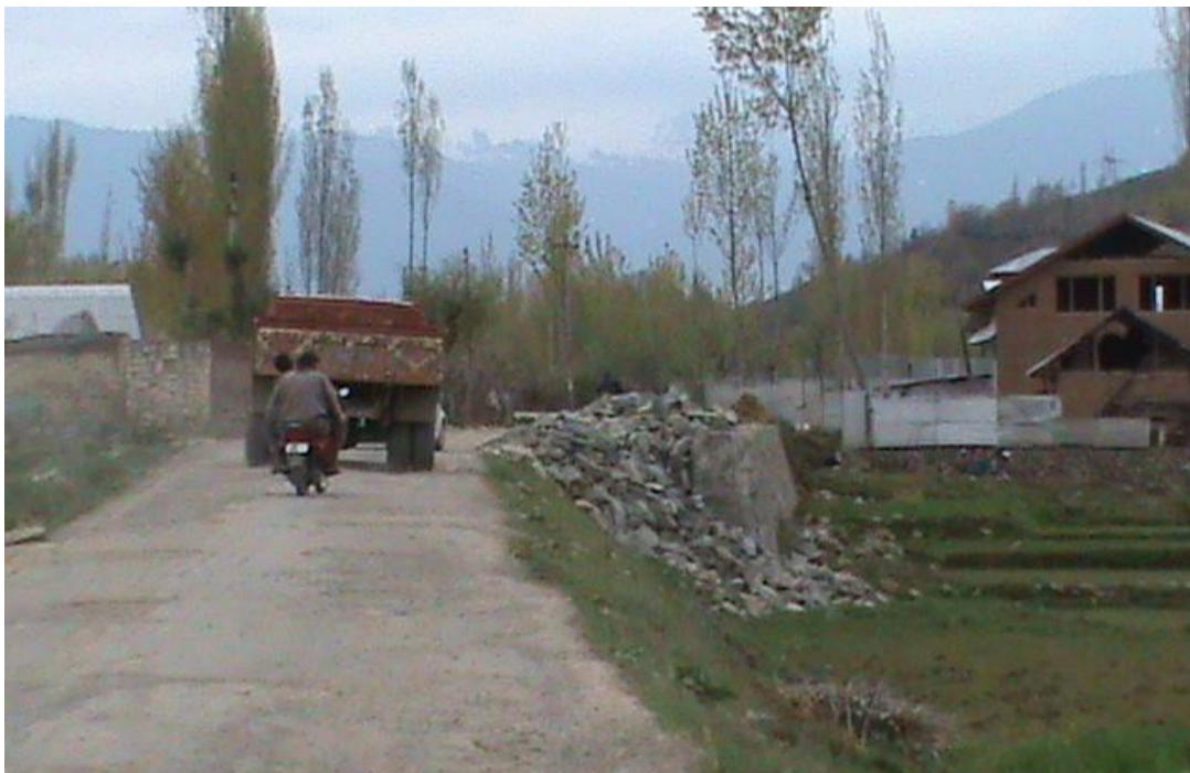
Spot at which the obstruction is caused in construction of Retaining wall and road
