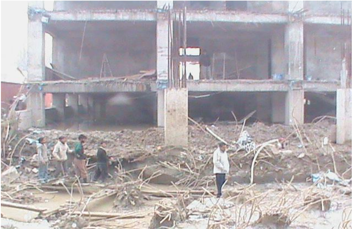
Cement concrete rafting in progress on backside portion of the main building
