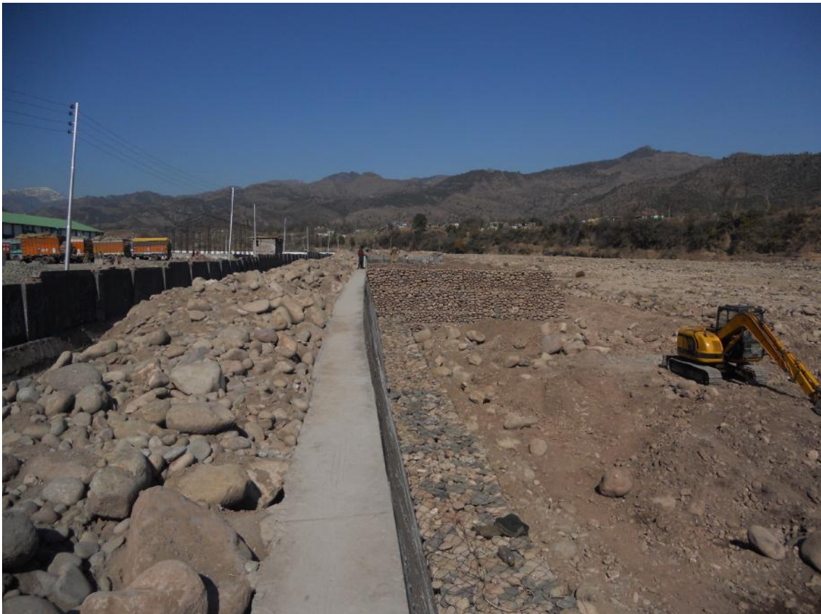
Flood Protection Work under progress on the eastern side of the premises
