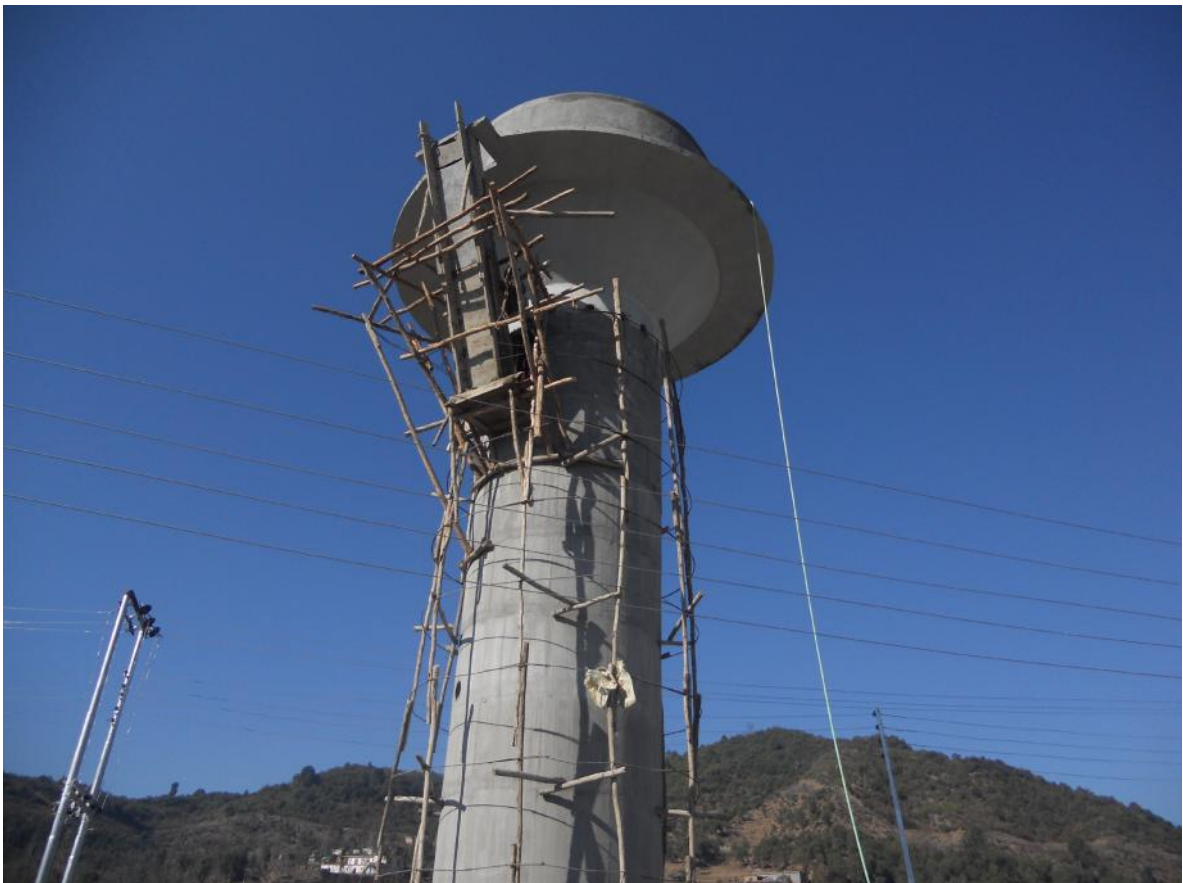
Overhead Tank of 10000 Gallons Capacity at TFC
