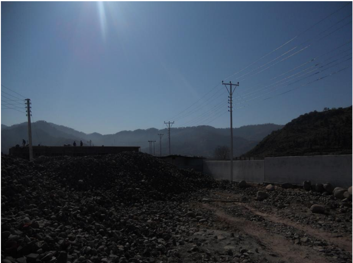
LT-HT Network laid on ST Poles
