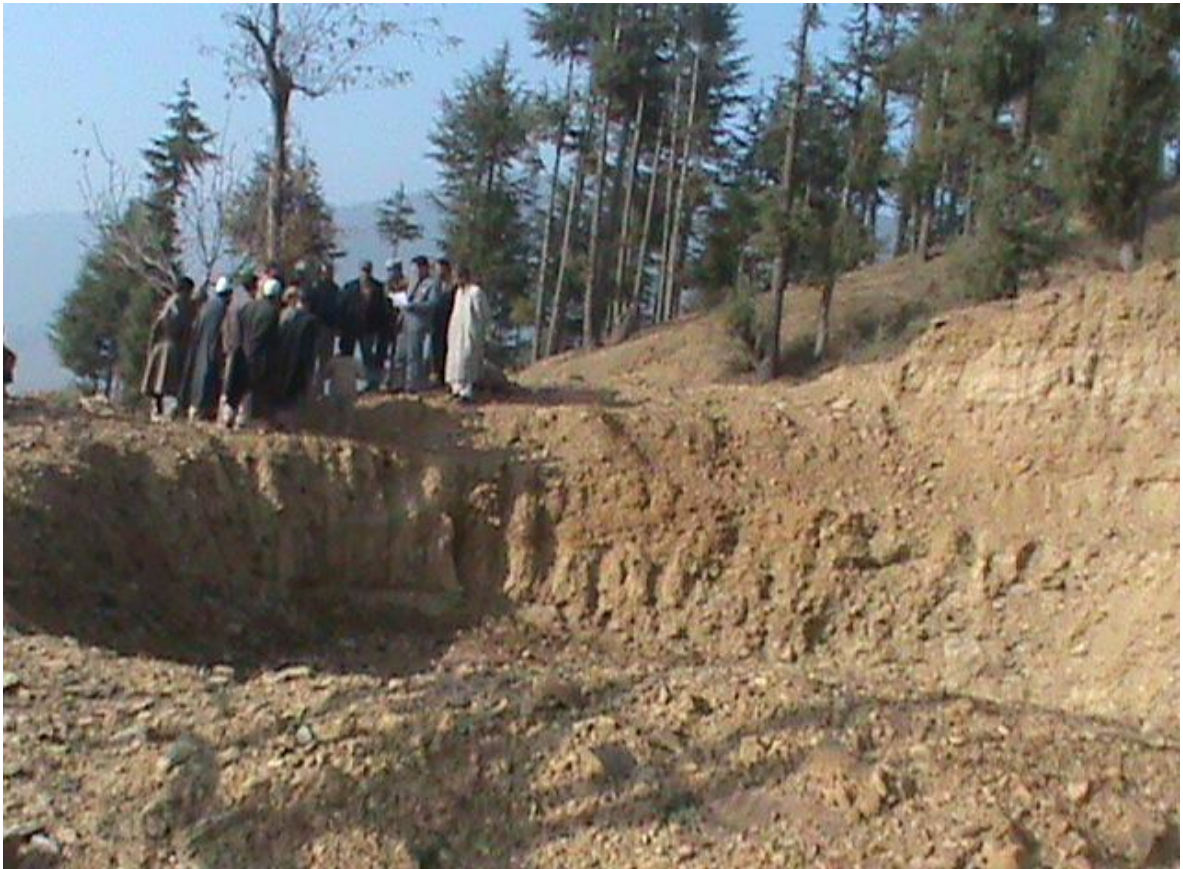
Earth excavation work for construction of new Service Reservoir for WSS, Batpora
