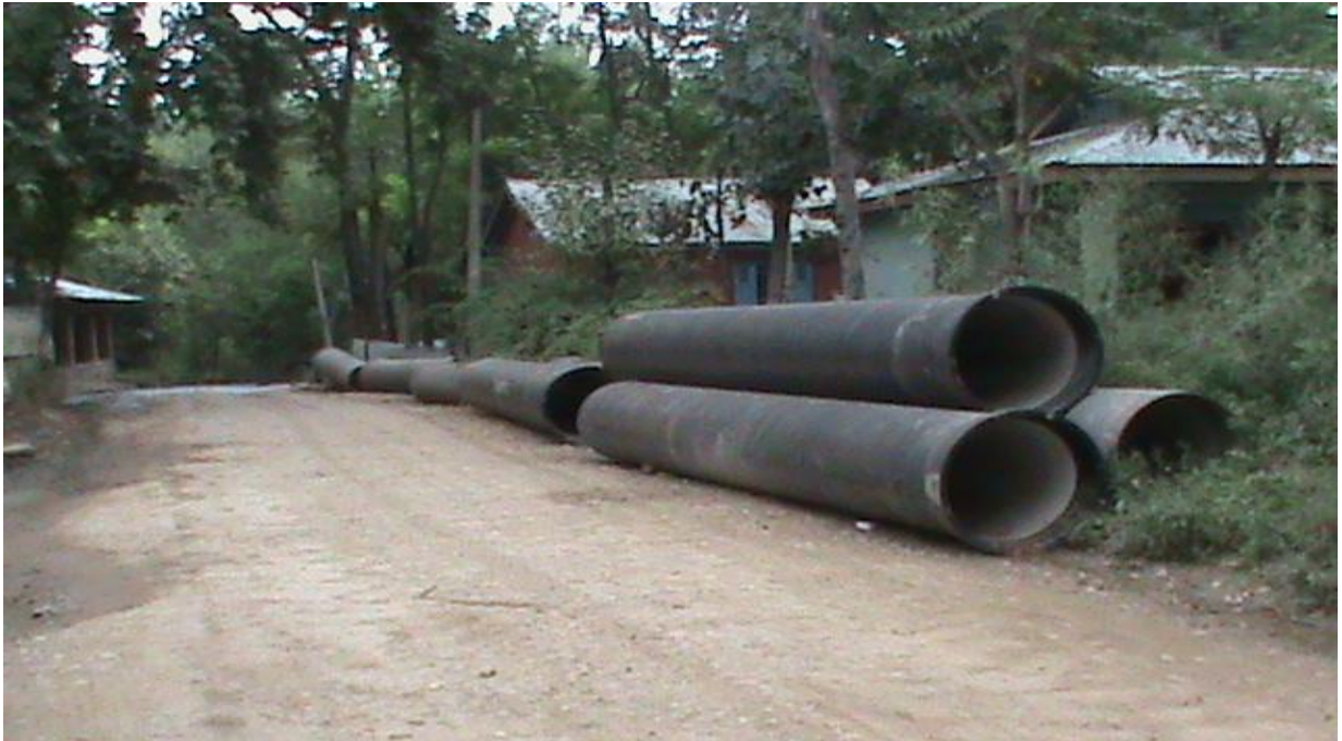
Pipes dumped at Brail - Parthan road stretch
