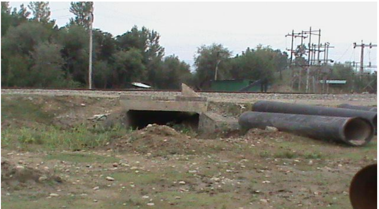
Railway track at Sebdan, (Budgam) where work for laying pipe under culvert is held up
