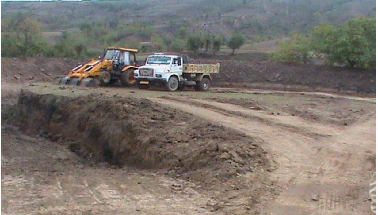
Site for construction of Treatment Plant at Parthan, earth excavation work in progress
