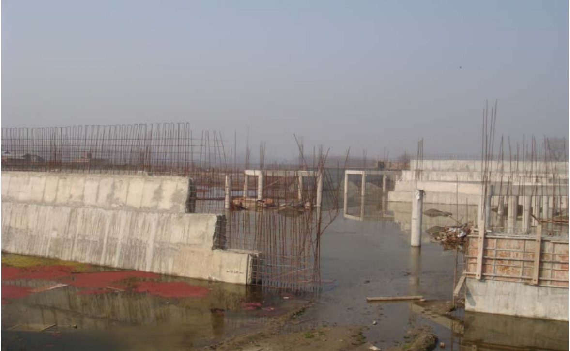
Water lodged construction site of STP at Noorbagh, Srinagar
