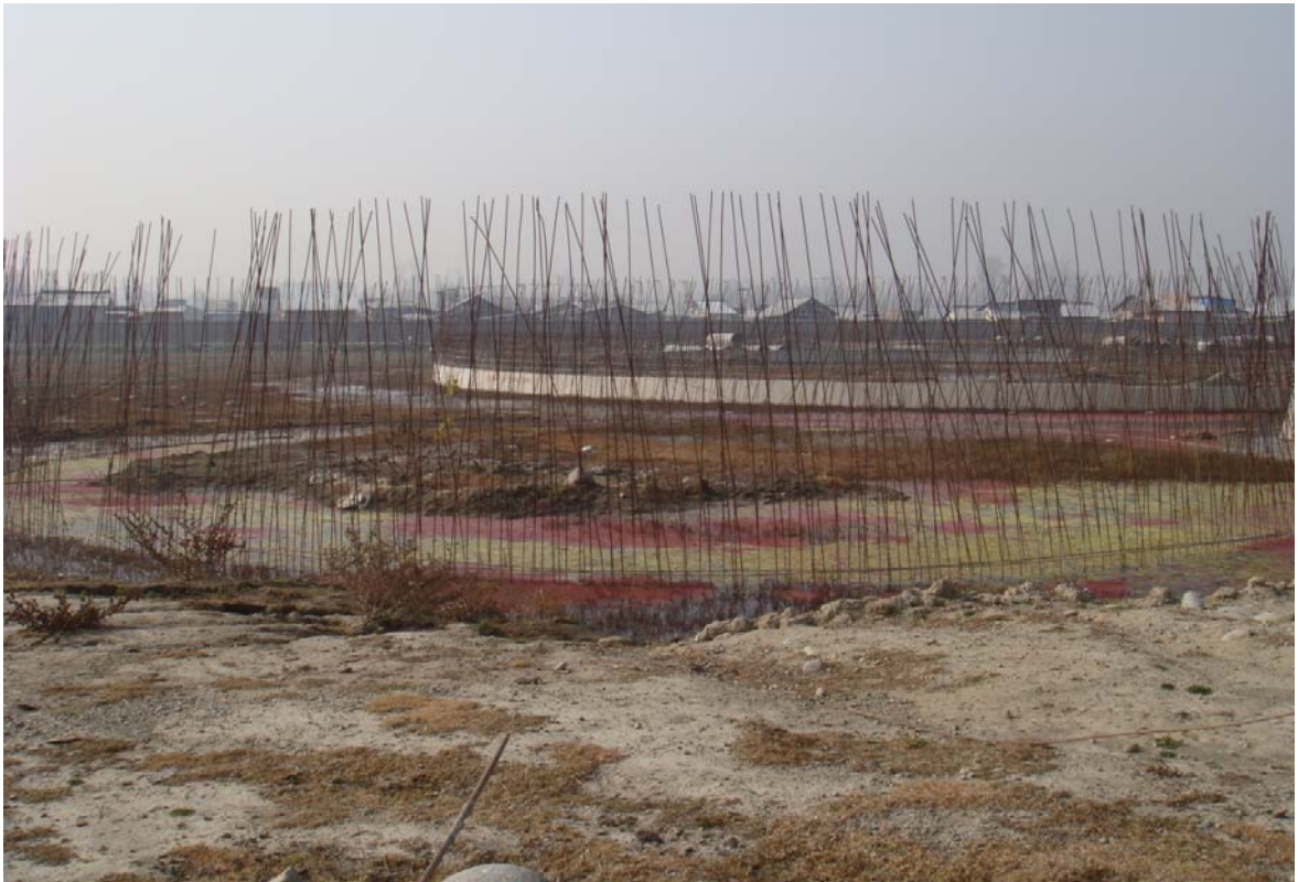
STP at Noorbagh, Srinagar
