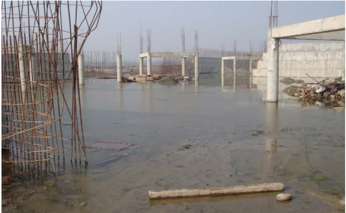
STP at Noorbagh, Srinagar in dilapidated condition
