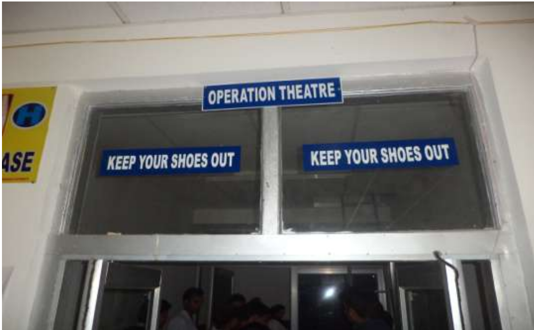
Almunium alloy door frames provided within the hospital building
