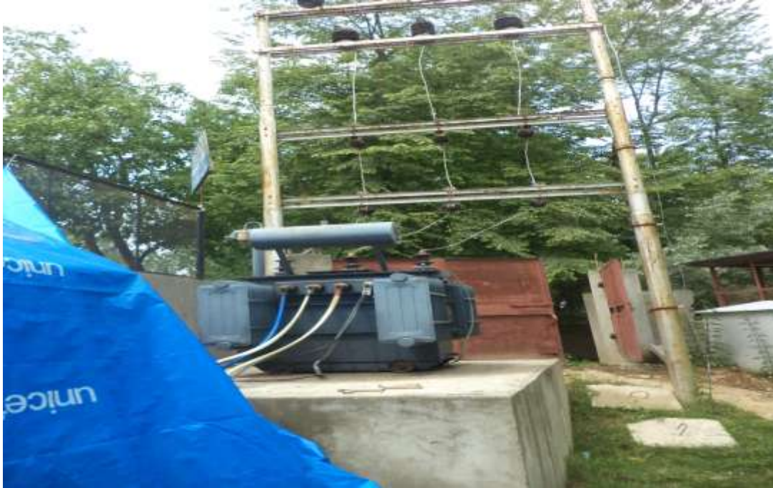
Creation of 630KVA capacity electric substation
